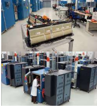
GM Worker Injured After Lithium-Ion Battery Explodes
